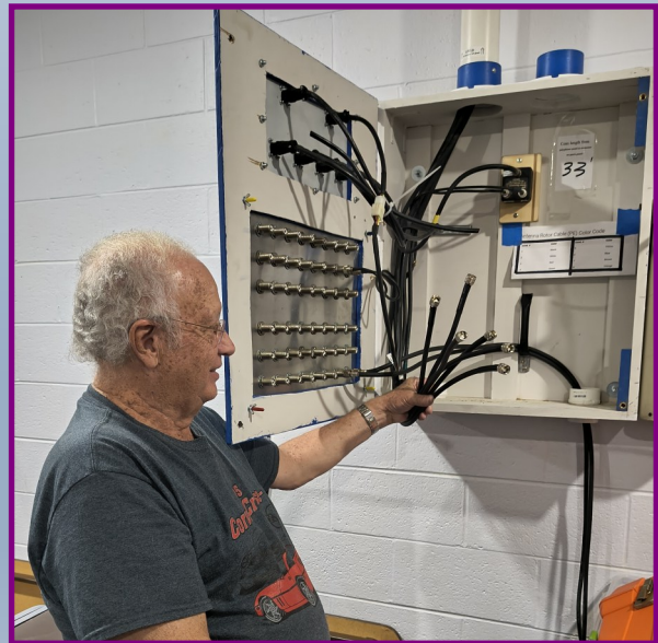
RF Coax trimmed with connectors to patch panel
