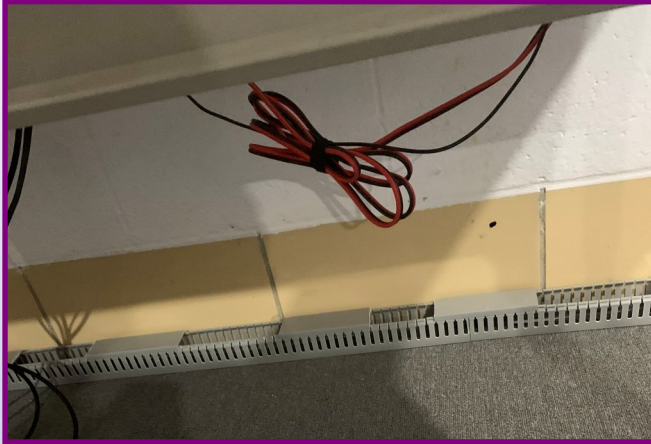
Cable Channel under Station 1
