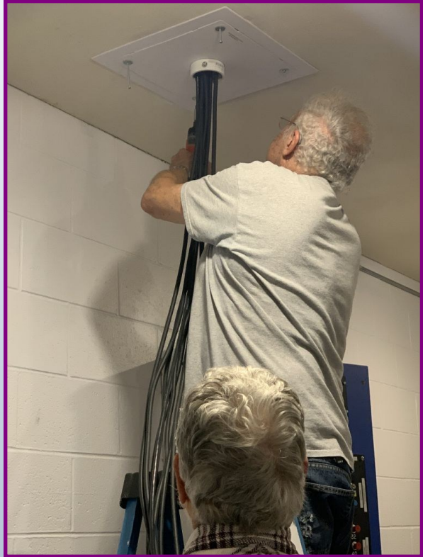
RF Coax in ceiling drop to patch panel
